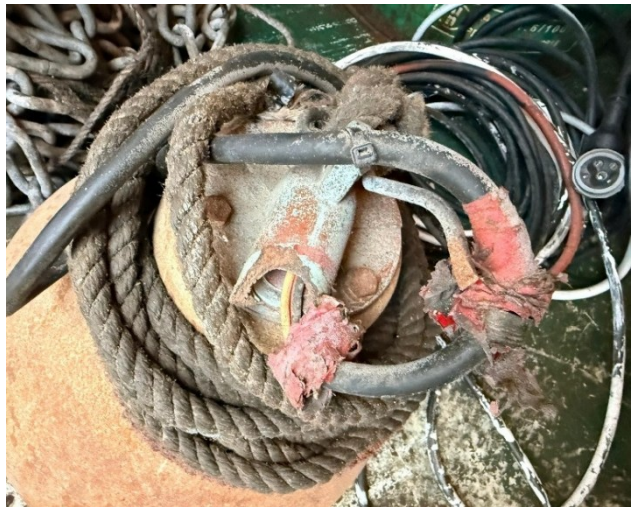
Unauthorised cable repairs and broken power cable gland
