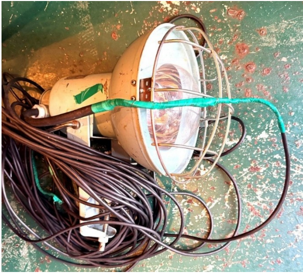
Improper cable connections Different specifications of cables connected
