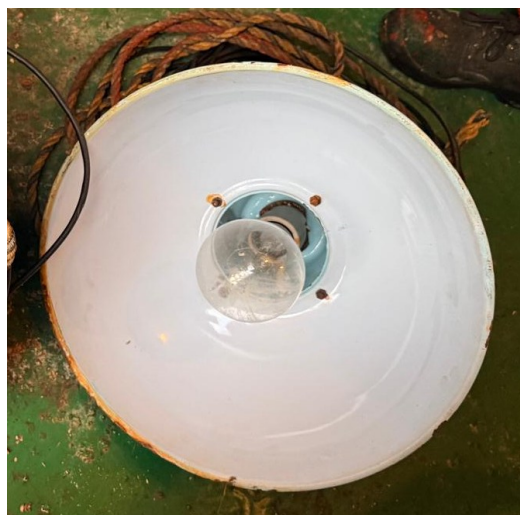
Missing safety guard
