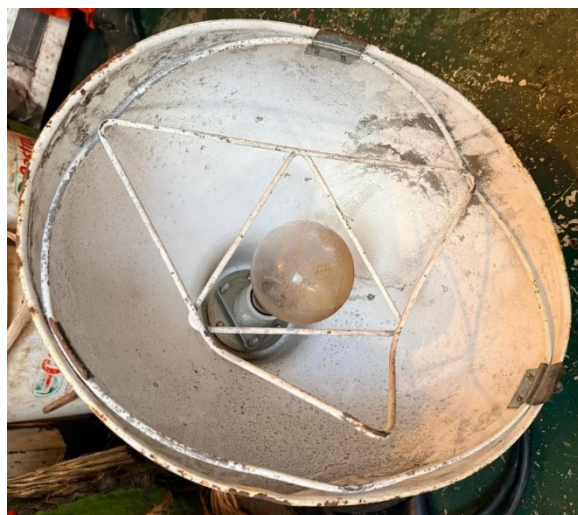
Damaged safety guard
