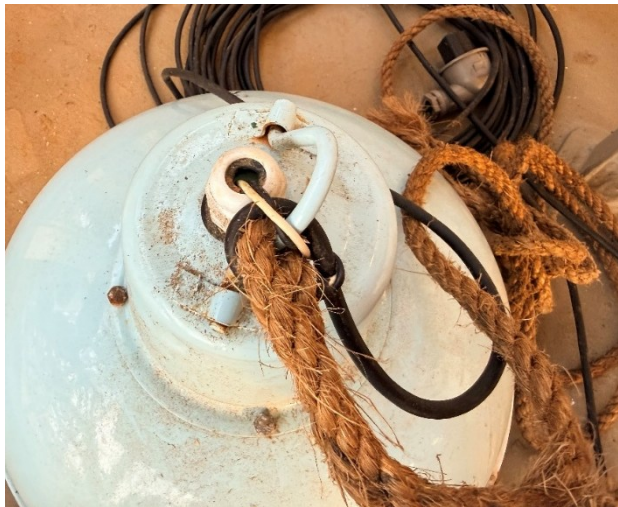
Power cable damaged and missing protective sheath Cable gland is loose
