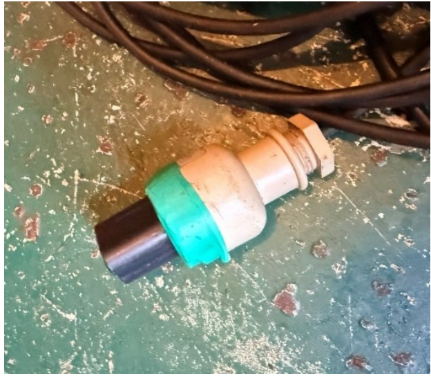
Damaged power plug with unsafe repairs
